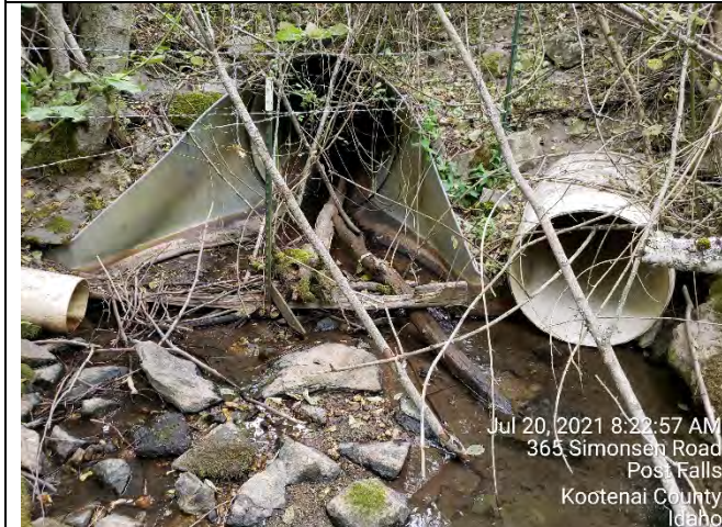
Inlet to Outfall #3LT
