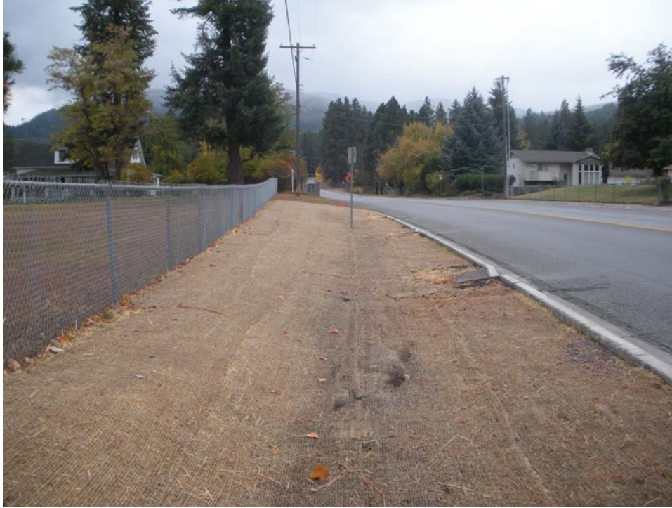
Photo 1: Spokane Street Drainage Improvements (10/23/12) New Swale with Jute Matting Upstream of Catch Basins/Outfall #6
